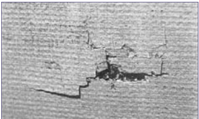
Figure 3.3-3. Damage on the inner surface of RCC panel 10-right from Atlantis after STS-45.
